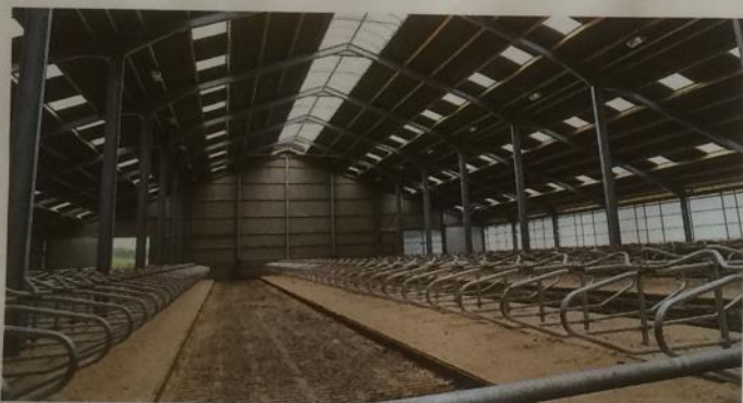
The 3.0m wide curved Airkoe light ridge was fitted to the 260-cubicle, 79m long, 39m wide building.
